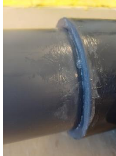
FIGURE 24: AN EXAMPLE OF A LEAKAGE PROBLEM IN THE PIPING SYSTEM
